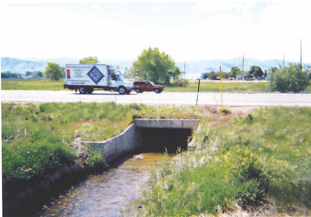
Boulder and Whiterock Ditch Culvert at BNSF Railroad Tracks (facing north, just south of Jay Road).
