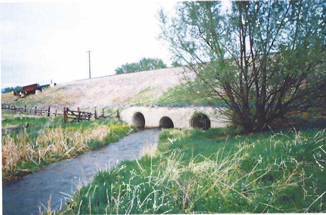
Culvert at Cottonwood No. 2 Ditch and Dry Creek Davidson Ditch crossing under BNSF tracks on south side (facing northwest).
